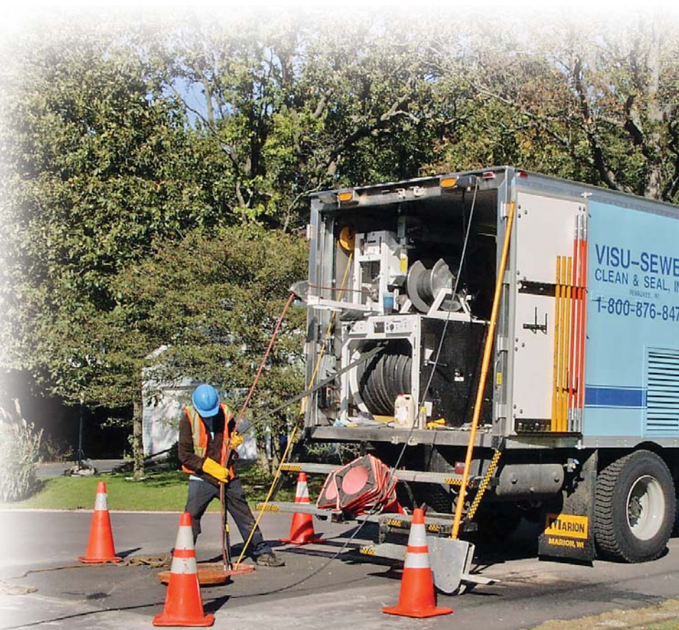
A technician from Visu-Sewer Clean & Seal Inc. starts an inspection of a sewer main in the City of Graettinger, Iowa, as part of the city's program to control inflow and infiltration.
